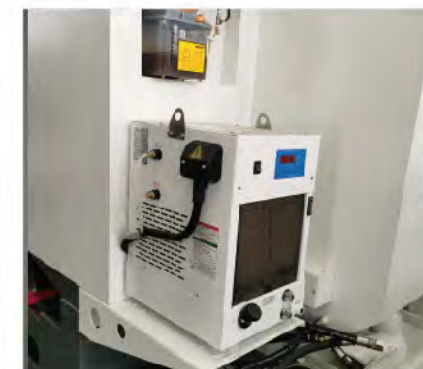
Spindle oil chiller
